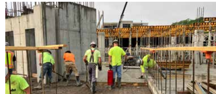
Future transit center on lower level of Vantage at Anderson Towne Center.
