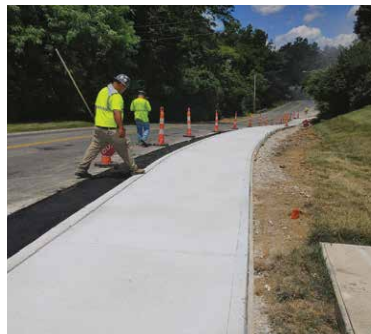
The Bartels Road sidewalk was completed before school was scheduled to start.
