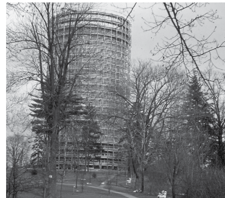
The Mt. Washington water tower under construction in 1939. It went into operation in 1940.
